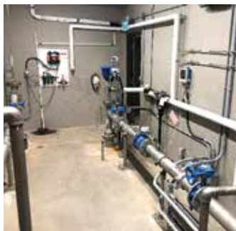
Milne PH - Treated water feed system out to the distribution
