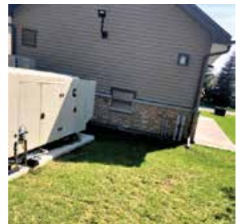
Milne PH Natural Gas Emergency Generator
