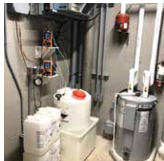
Milne PH chlorine feed system
