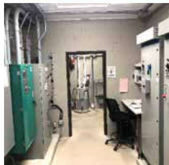
Milne PH - Electrical control room
