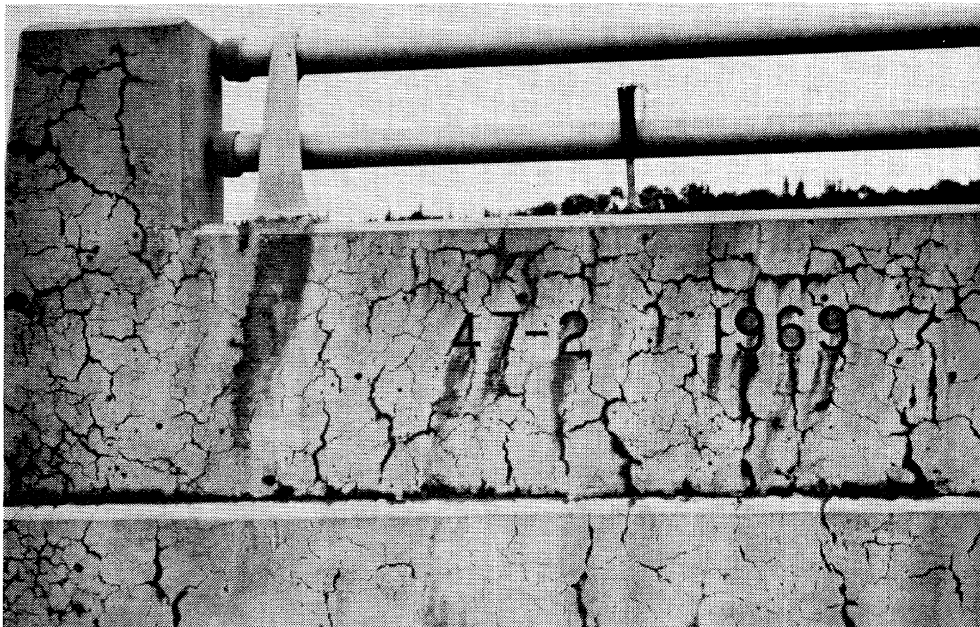
Figure 14 Alkali-silica reaction, Englehart River Bridge, Hwy. 66, built 1969. Cracking is due to a reaction with Precambrian chert which was waste rock from a local mine.
