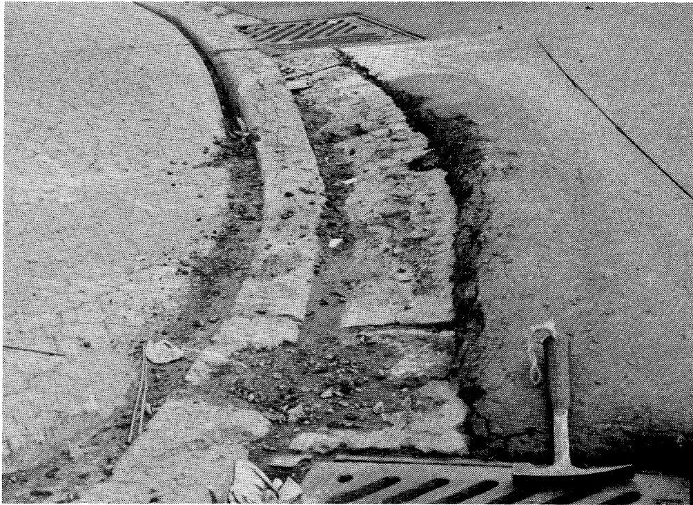
Figure 3 Alkali carbonate reaction, Lancaster. Expansion of sidewalk from left to right has pushed curb about 6 cm into pavement, causing shoving of the asphalt.
